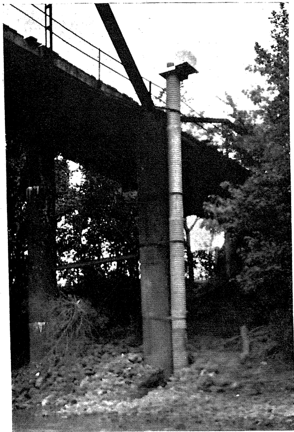
View of recording gage on Sac River near Collins, Mo., which gives a continuous graphic record of the stage of the river. (Furnished by West Missouri Power Co.)
